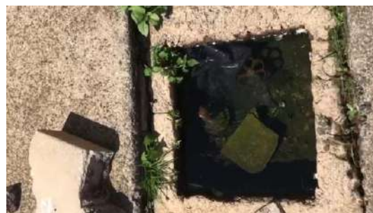
Flooded drain due to the leak on the hospital premises
