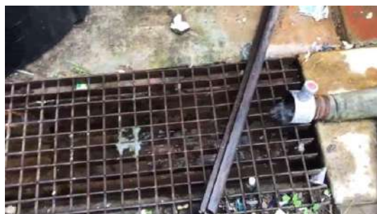
Water leak into a drain on the hospital premises
